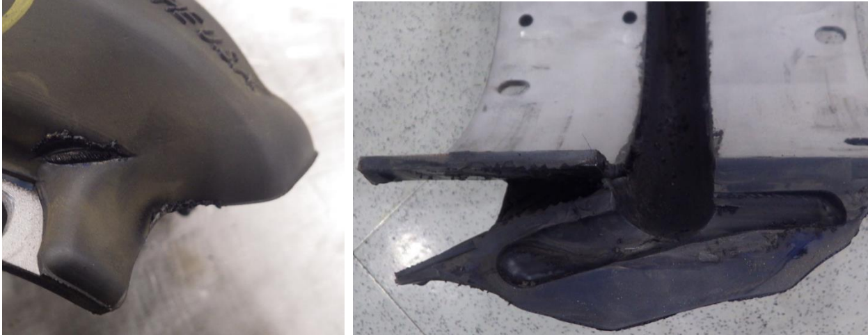
Figure 4: Typical tearing patterns at the element split as a result of excessive misalignment, torque, or vibration.
