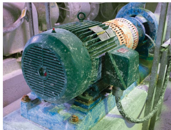
Because of the wet environment in the mill, Essity officials point to the Inpro/Seal non-contact labyrinth seals at both ends of the motor as another key to the quality of the ABB’s Baldor-Reliance IEEE 841XL motor.
