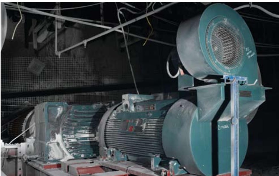
A 700k MagnaGear XTR reducer is connected to a 700 HP Baldor•Reliance® Mining Industry motor in this underground mining application. The tough construction, plus the bearing and seal designs of this motor, makes it ideal for harsh mining conditions. The blower keeps the motor cool across its entire operating speed range.
