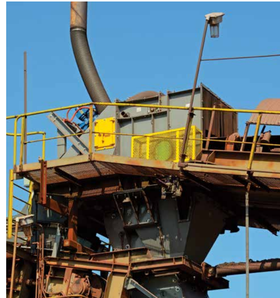
The Toledo Docks facility has run more than 3 million tons of ore since the installation of the Baldor•Dodge® Hydraulic ISAF (located behind the yellow guard) on its new high-flow shoot. Because of the bearing's reliability, ease of installation and expected ease of removal, company officials expect more Hydraulic ISAF units will be installed in the future.
