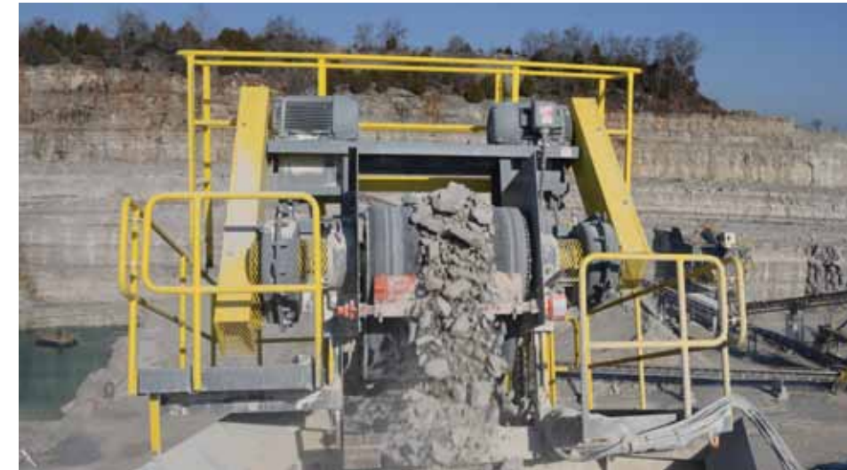
Process Machinery relies on Baldor's System-1 group, a team that facilitates the design, quotation and order processing of multiple products for project support. The System-1 group also ensures that all of the packages and other components are delivered on time and in the right order.
