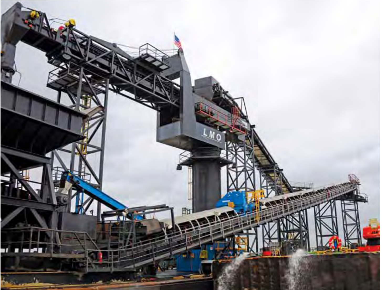
The Louisiana Mid-Stream One (LMO) is a unique barge-mounted conveying system with quality control features not found in other midstream loading operations, including a magnet, mechanical sampling system, belt scale and water drainage. The LMO can simultaneously feed and combine product from multiple barges to meet quality specifications, enhancing the quality of export coal.
