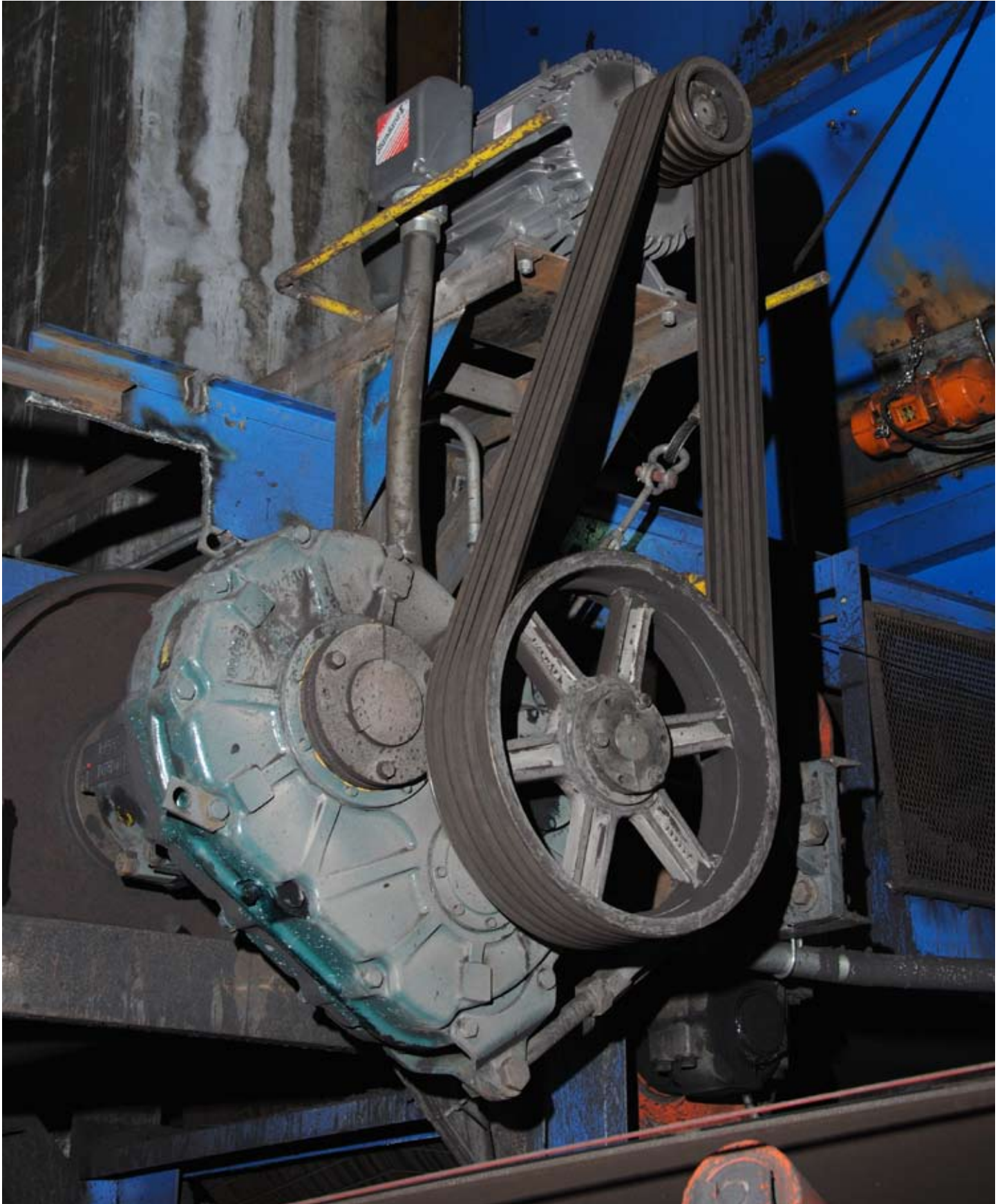
A size 10 Baldor•Dodge TXT, Baldor•Dodge V-belt drive and 75 HP Baldor•Reliance motor were selected to power one of the largest conveyors at the Mesabi Nugget plant. (Please note that this equipment was not running, and the guards were removed for photographic purposes.)
