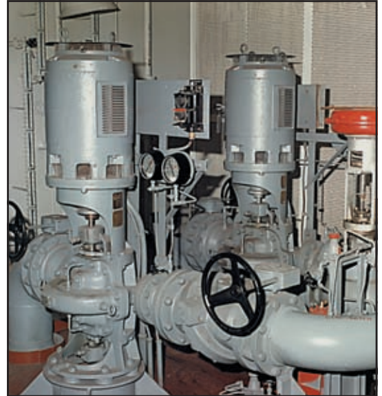
The pumps of this fresh water circulation system are powered by our 50-HP, 1800-RPM vertical P-base motors.
