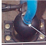
Figure 6-1 Block Heater Hoses
