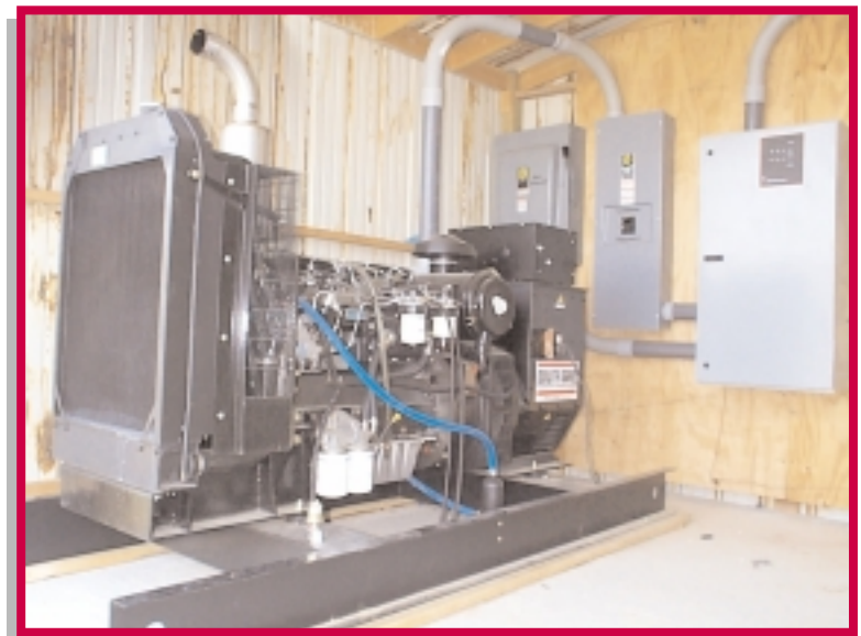
DLC100 connected to Baldor 400 amp ATS
