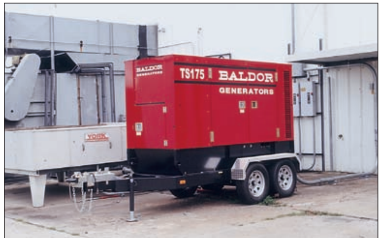
Baldor TS175T used in a load-shedding application. The 100 ton air conditioning unit is taken off the utility grid during peak consumption and switched to the genset.
