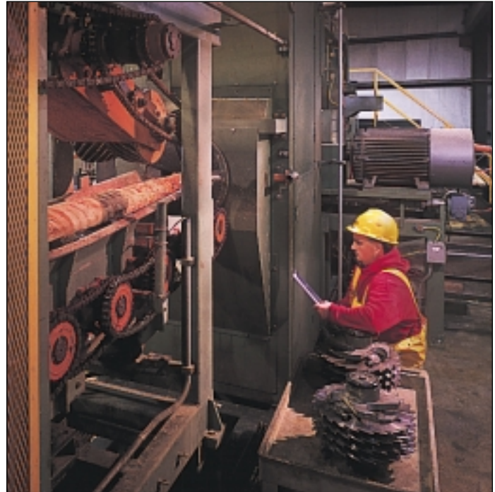
A Baldor 500 hp, medium voltage Chemical Processing Motor (pictured at the back end of the machine) and Series 22H Line Regen Vector Control run this chipping machine at a North Carolina lumber mill. High performance and reliability are the hallmarks of this Baldor motor, running in multiple shifts, under high-torque demands, exposed to sawdust and other airborne contaminants.
